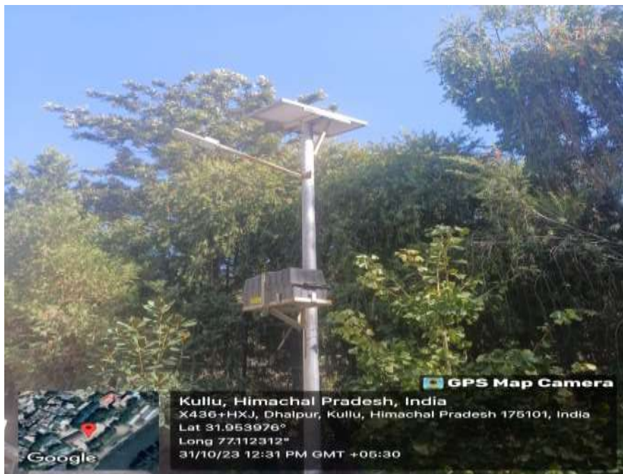
Figure 9: LED Street Light
