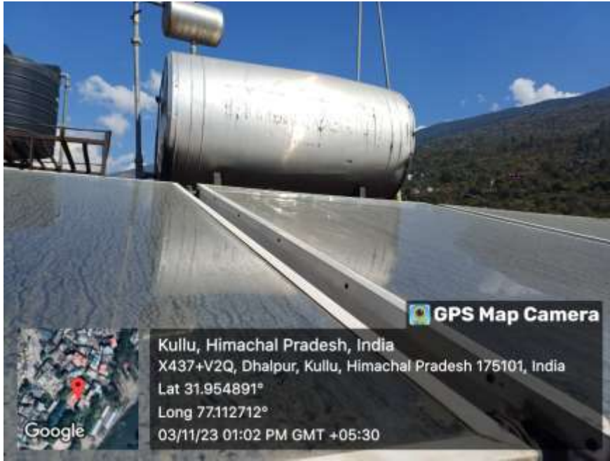
Figure 6:Solar Water Heater-3
