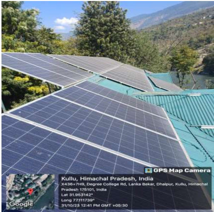
Figure 1: Solar Plant at Arts Block (28 kWp)
