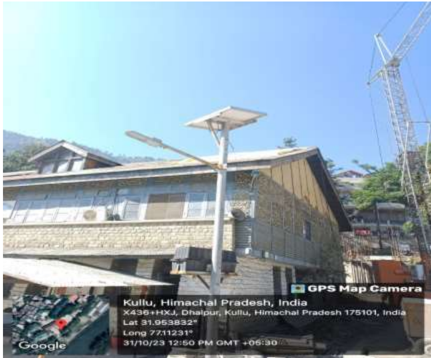
Figure 8:LED Street Light
