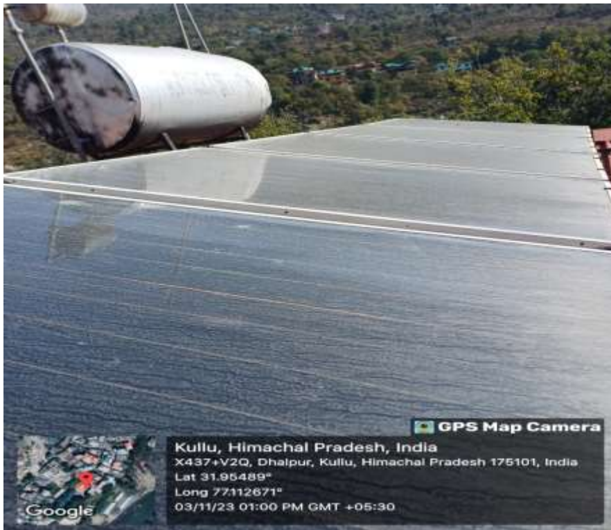
Figure 7:Solar Water Heater-4
